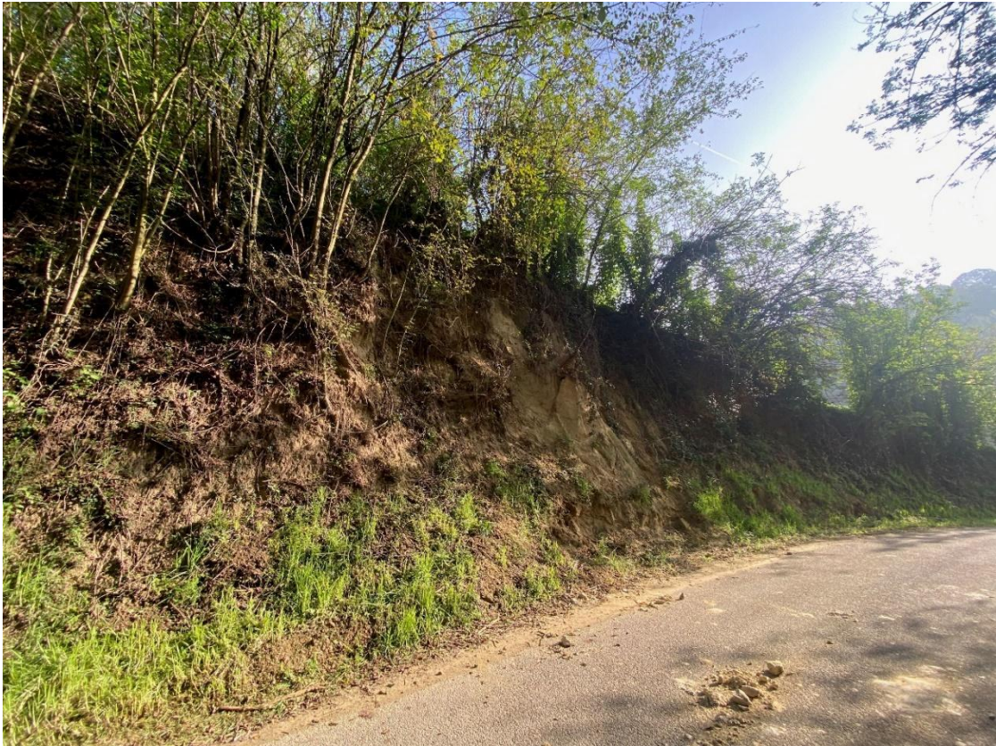
Figure 13: Wall subject to small-scale collapse in the Moncucco area
